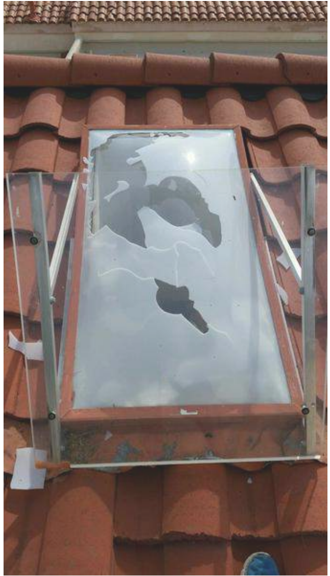
Broken skylight presents risk of water entry and glass shards entering house.
