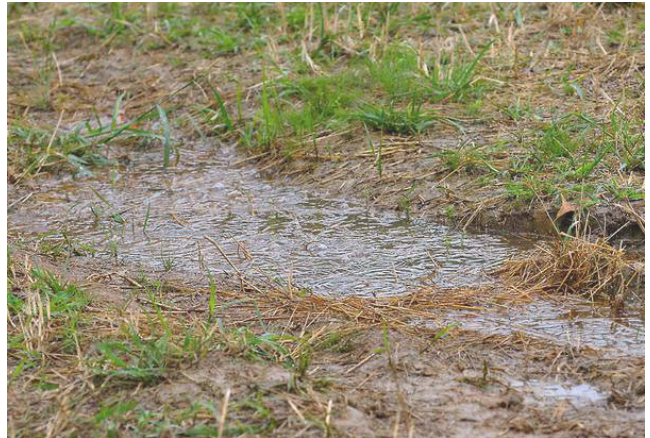
Water pooling in yard; recommend drainage
