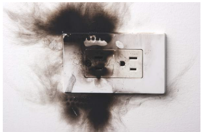
Scorch marks on cover plate
