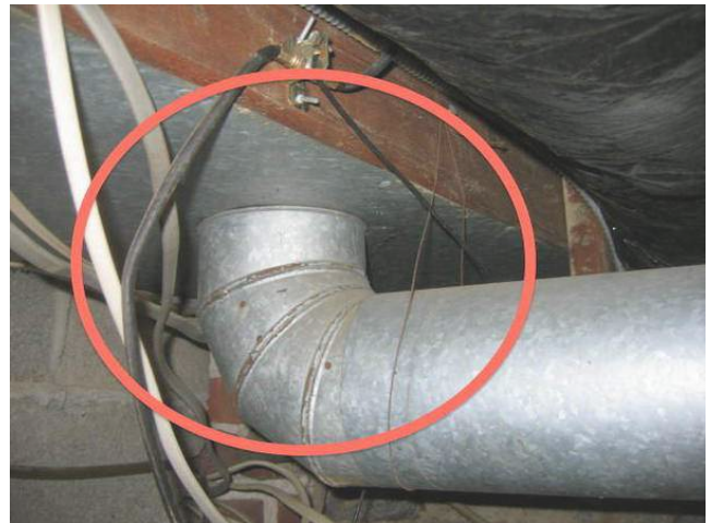
Loose connection; recommend sealing.
